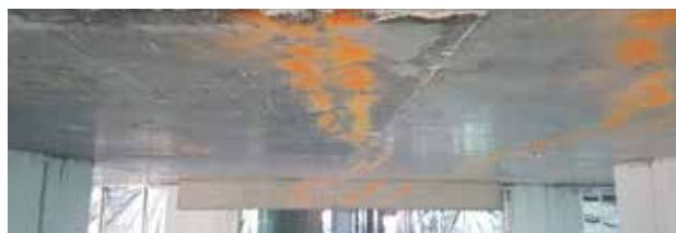
Formwork residue and concrete debris often present uneven fixing surfaces which are not made good prior to wall installation.
